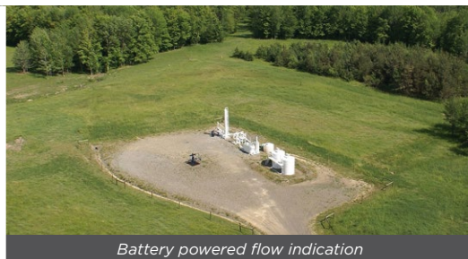
Battery powered flow indication
