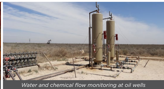
Water and chemical flow monitoring at oil wells
