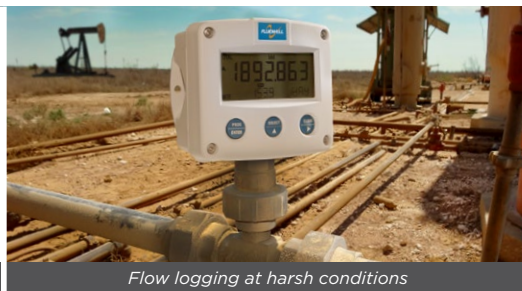
Flow logging at harsh conditions
